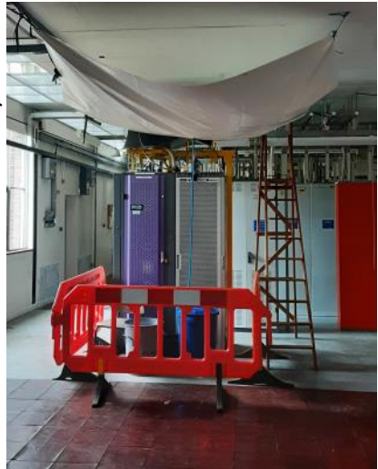
Water Leak Sorted!
